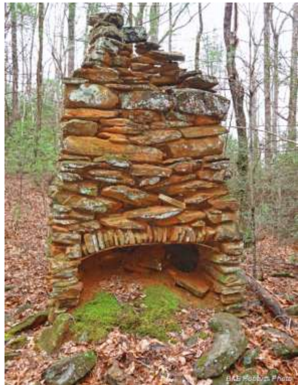
Chimney with collapsed top (Rocks stained from the clay chinking)
